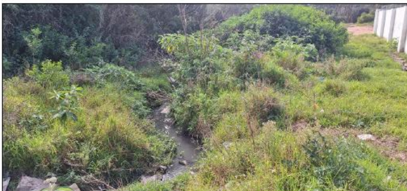
Plate 9: A photograph taken of the UC/B 2 system showing the eroded channel and alien vegetation.
