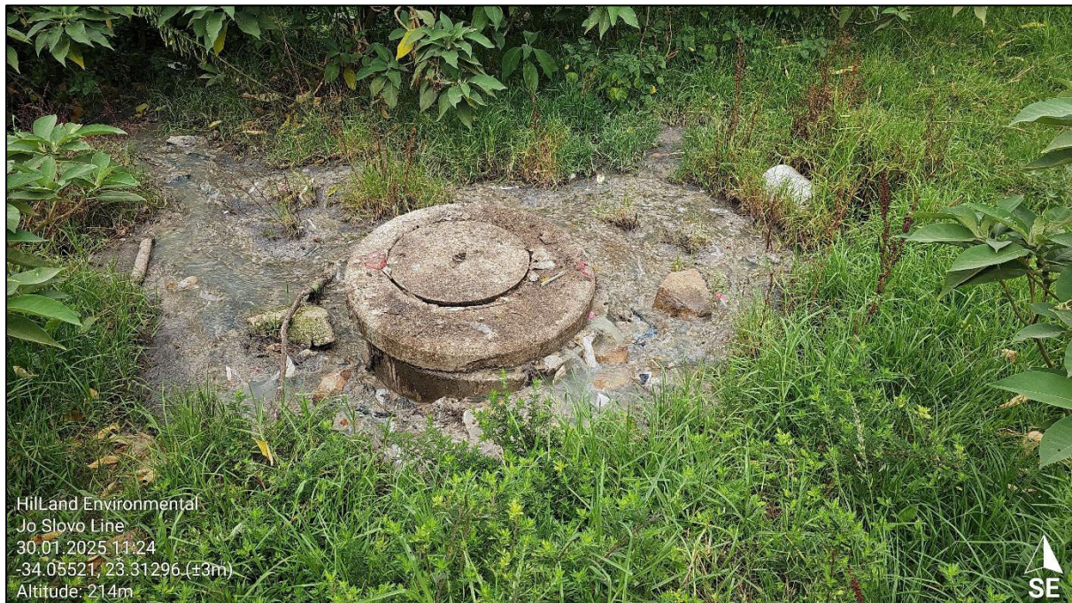
Figure 2: Overflowing manhole of raw sewage supplied by HilLand Environmental
