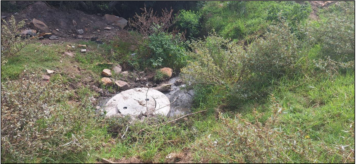
Plate 3: A photograph taken of the overflowing sewer manhole which directly flows into Rip 1.
