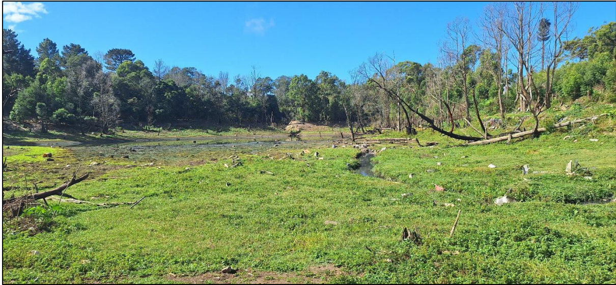
Plate 10: A photograph taken near the confluence UCVB 1 and 2 showing the old dam which has a hole in it
