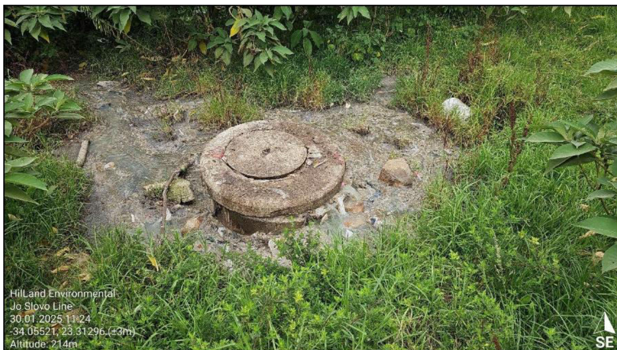
Figure 2: Overflowing manhole of raw sewage supplied by HillLand Environmental
