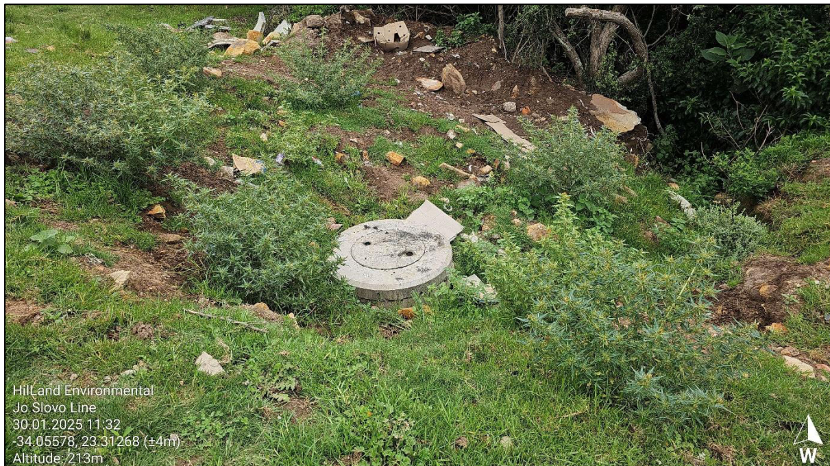
Figure 3: Sections of line have been undercut and eroded which requires repairing.
