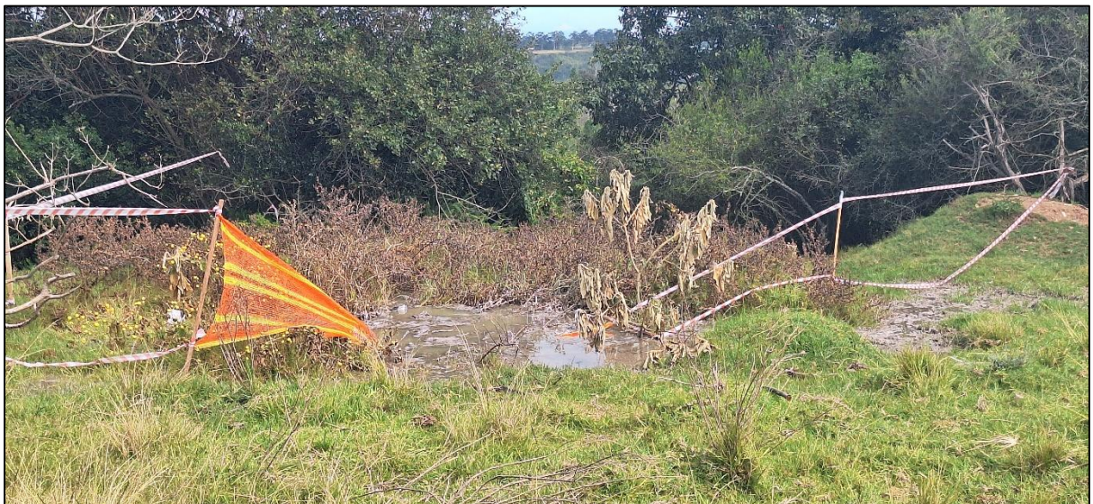
Plate 4: A photograph taken of the overflowing sewer manhole which directly flows into Rip 2.
