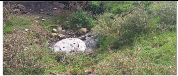
Plate 3: A photograph taken of the overflowing sewer manhole which directly flows into Rip 1.
