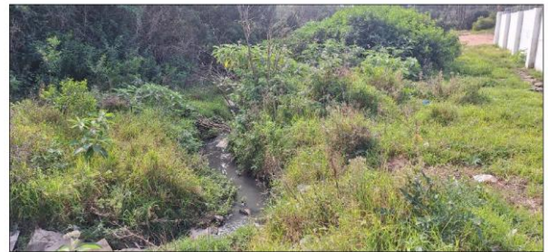
Plate 9: A photograph taken of the UCVB 2 system showing the eroded channel and alien vegetation.
