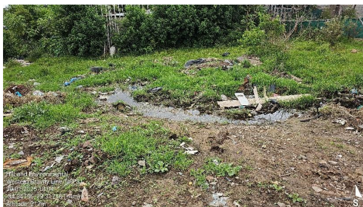
Figure 9: Leak at western gravity line to PS1
