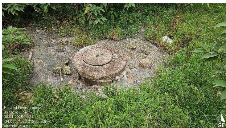
Figure 8: Overflowing manhole (JoSlovo line) – full photographic records attached to Appendix C
