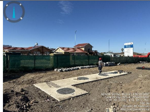
Underground fuel storage tanks.
