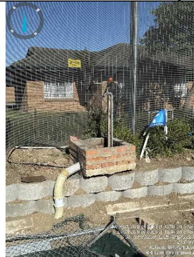
Potable water tap with silt trap connected to municipal infrastructure.
