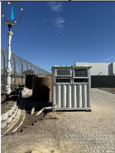
Construction phase ablution facilities connected to municipal infrastructure.
