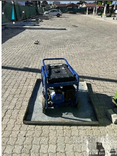
Suitable drip tray used for generator.
