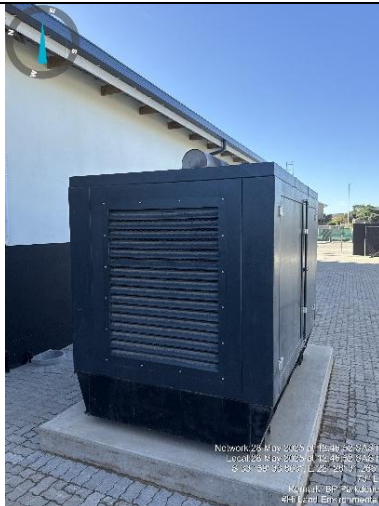
Backup generator for the operational phase has been installed.
