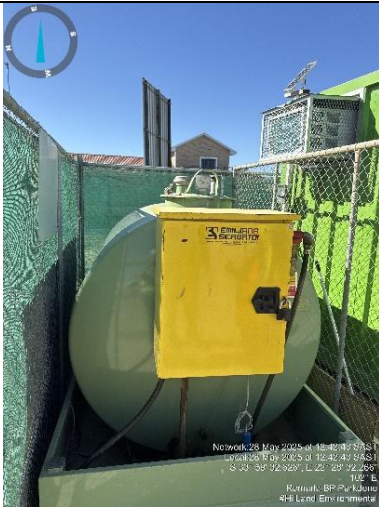
Temporary fuel storage (for construction phase) with bunding.
