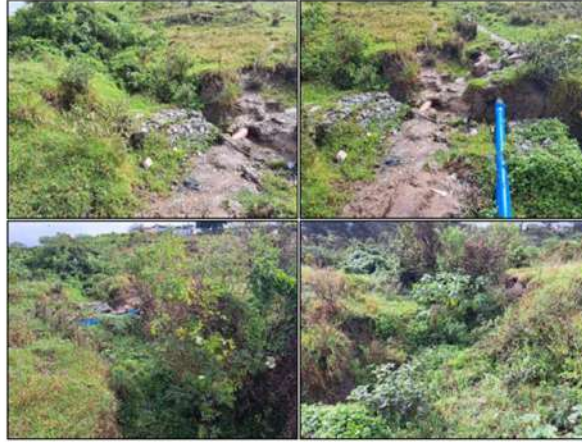
Figure 12: Photographs at Site 77 illustrating the exposed sewage pipeline, eroded bed and banks and incised channel.
