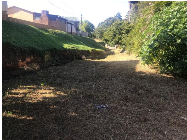
Figure 12. Most eroded bank on the left-hand side around the 110m cross section.
