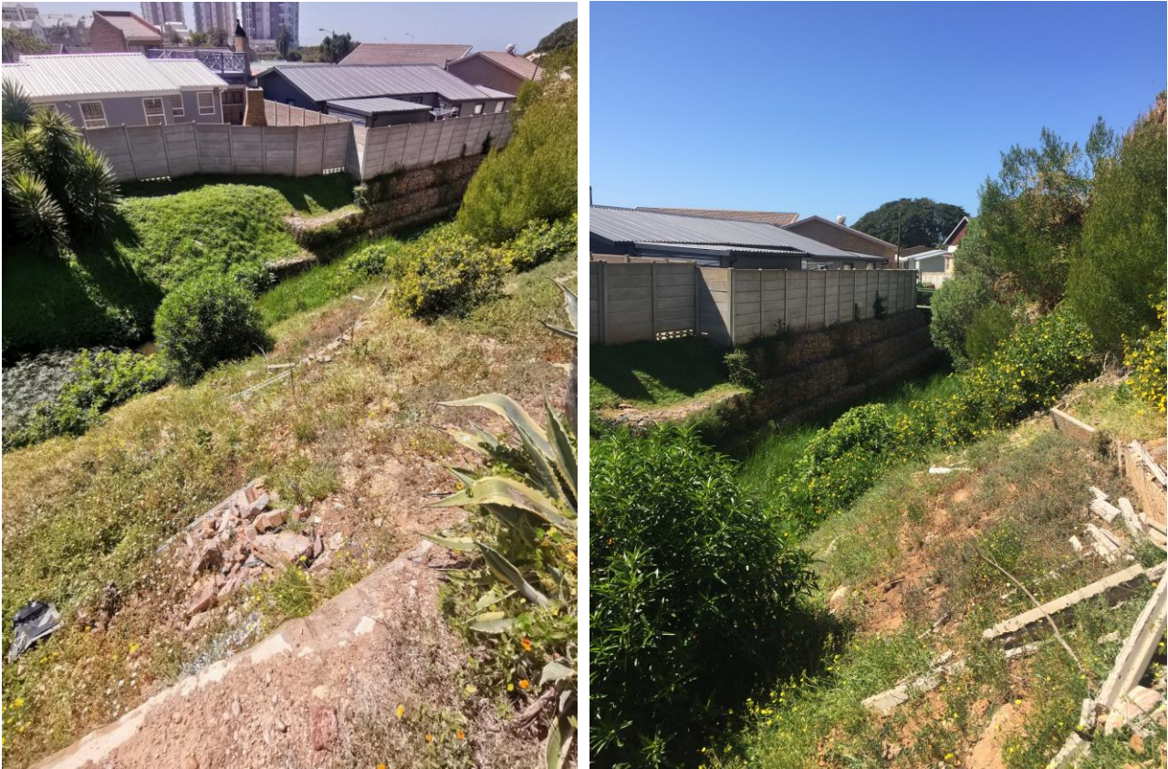
Figure 3-4: Boland Park embankment erosion
