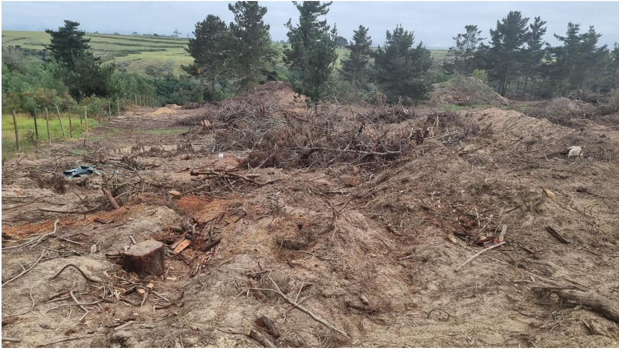
Photo 2: The extent of soil disturbance and plant debris indicate that the area was cleared by heavy machinery.
