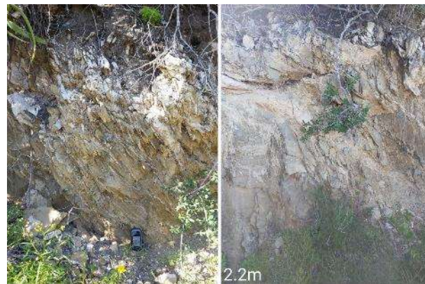
Plate 6. Examples of the shale exposed in the profile of road cutting shown in Figure 5. Note that the shale is nearly vertically bedded in places, showing significant folding / faulting / deformation. The GPS unit is 10cm long and the profile on the right is about 2m in height. Calccrete caps the shale in several places."
